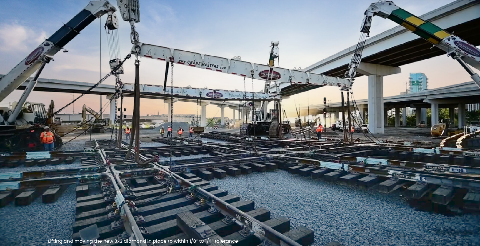
Lifting and moving the new 3x2 diamond in place to within 1/8" to 1/4" tolerance
