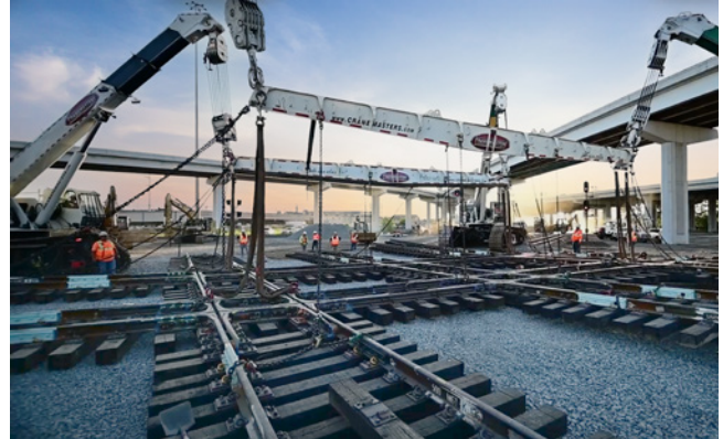
Cranemasters dismantles the old Tower 55 diamond in Fort Worth, TX, and lifts the new diamond—a massive 3x2, 126'-2" by 93'-9" 187,000-pound interlockings—and moves it in one piece in just 15 hours.
